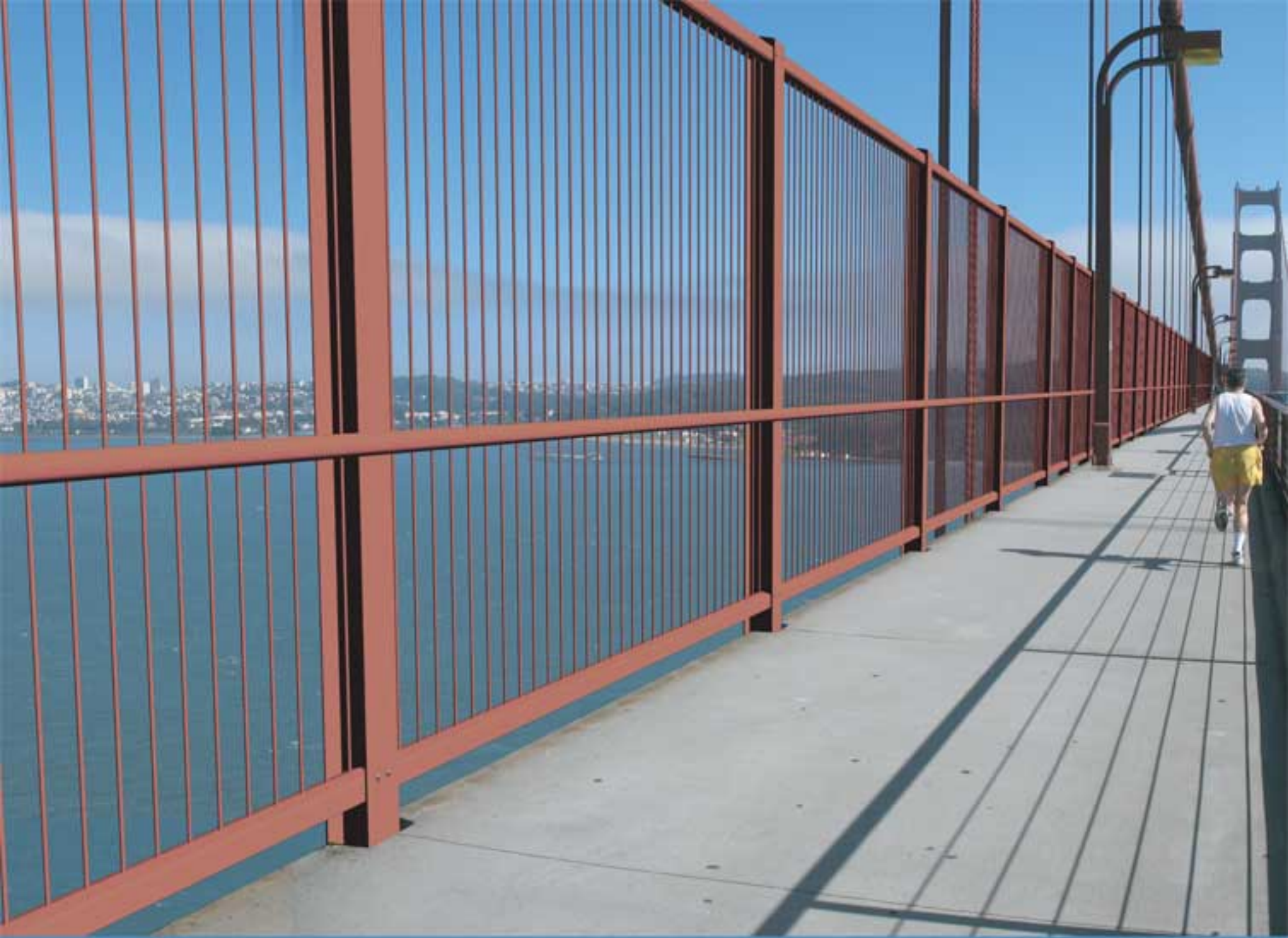
Alternative 2A - Replaces 4-foot handrail with 12-foot-tall vertical system Sidewalk View South
